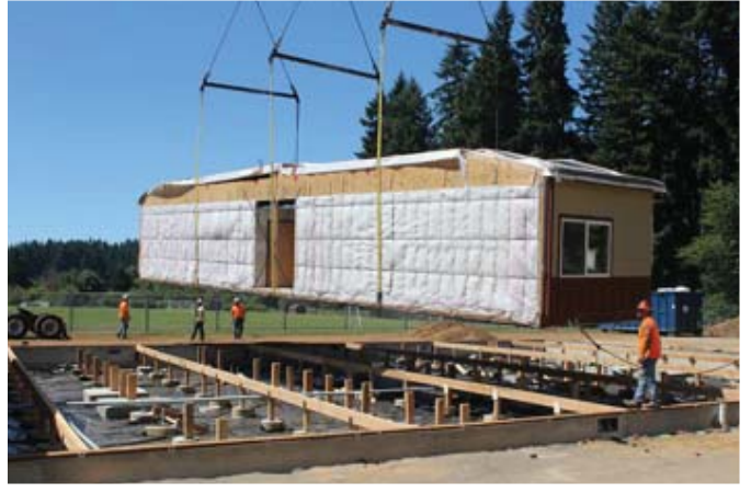
One of 11 sections that compose a new modular classroom building is swung into place on the Pleasant Valley campus Thursday, July 25.
